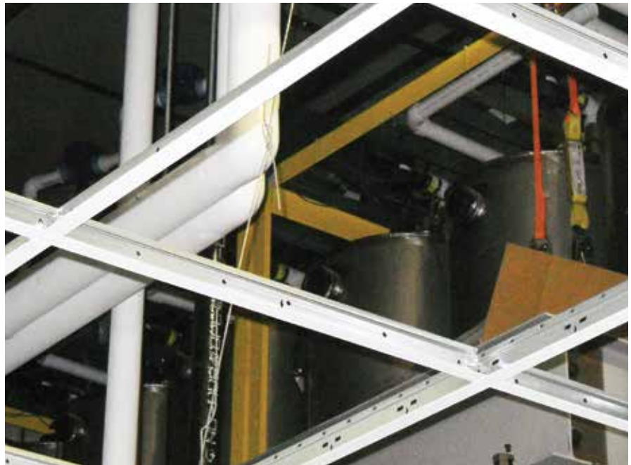
View of the vacuum center installed above the kitchen
