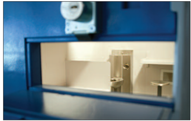
A "combi" vacuum plumbing system at a state prison.
